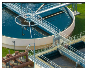
Effluent Treatment Plant
