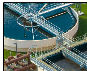
Effluent Treatment Plant
