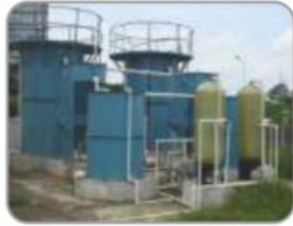
Effluent Treatment Plant
